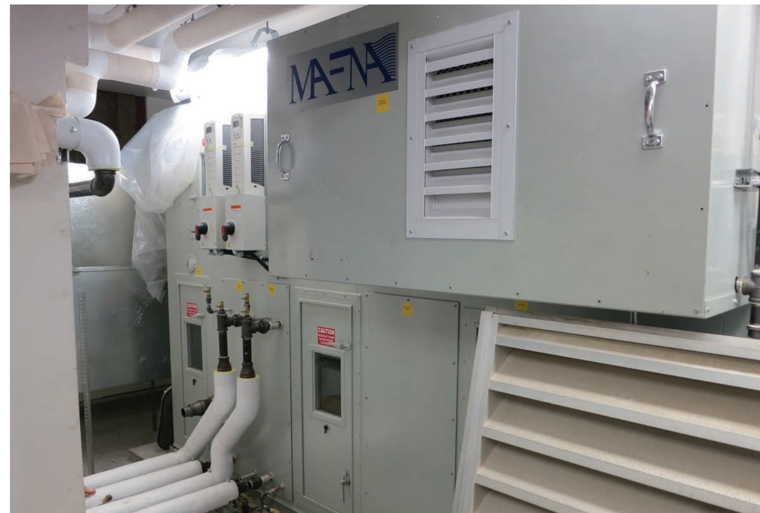
Our Collections Matter may examine tools that can assist heritage institution in optimizing HVAC systems to identify energy savings. Photo — © Government of Canada, Canadian Conservation Institute. CCI 128879-0005
