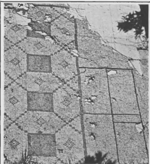
Fig. 9 - Mosaic transferred to reinforced cement. Badly insulated steel bars rust and slowly split the cement and the mosaic
