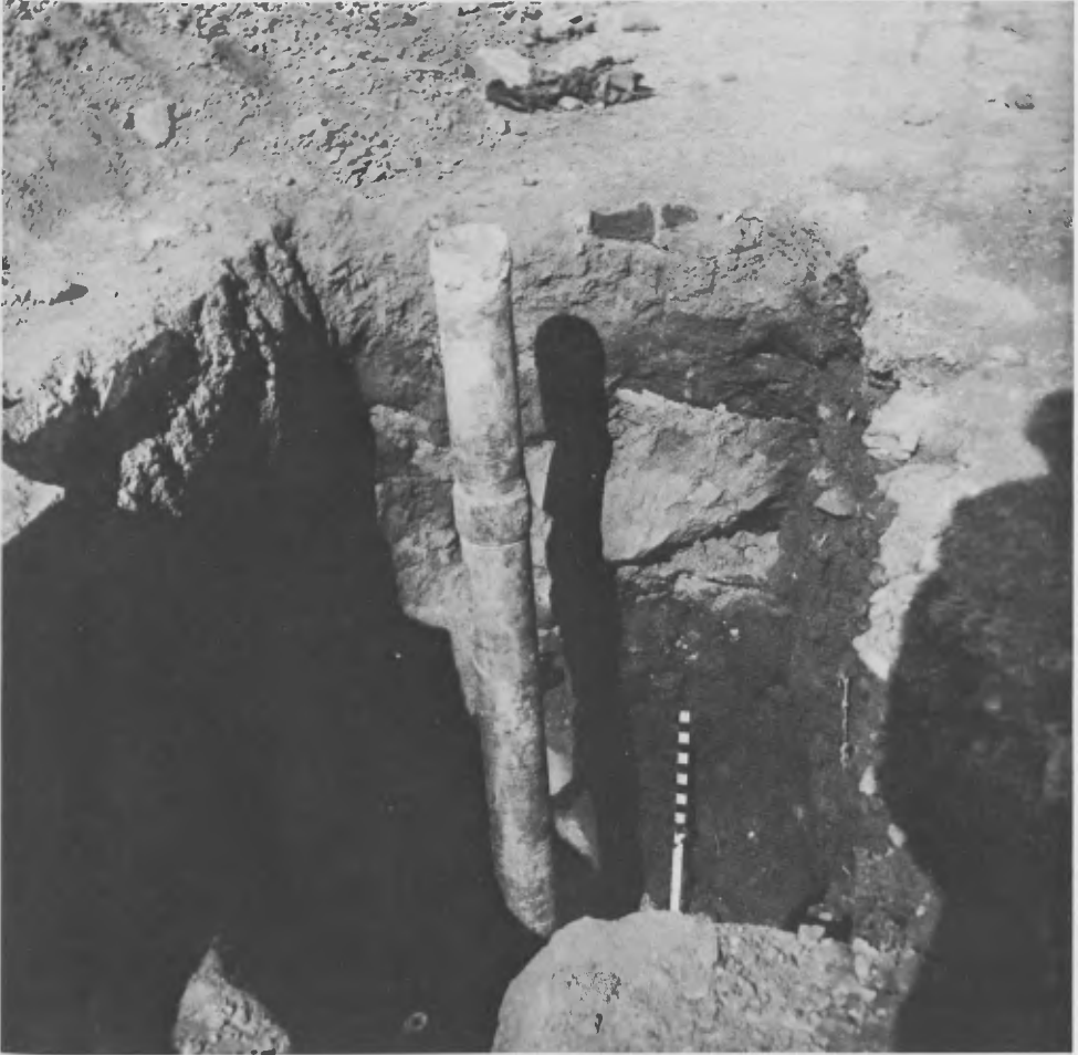
Fig. 7 - The Qutb Minar: A casing pipe used in grouting where the overburden was of loose material
