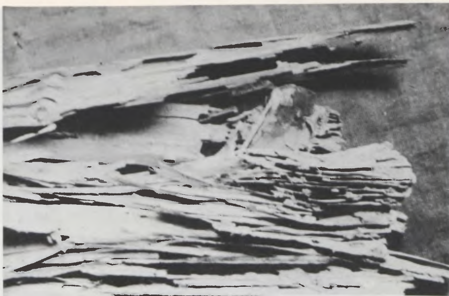
Figure 18. Termite-damaged wood with laminated appearance.
