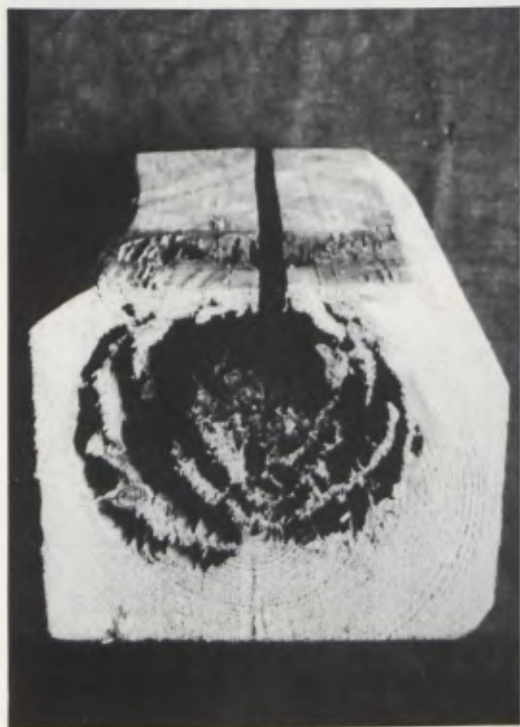
Figure 19. Beam hollowed out by termites.
