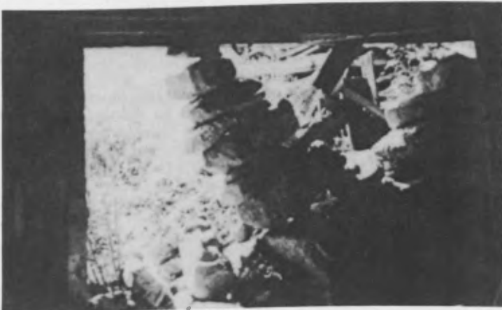
HARRISVILLE, N.H.: Ruined barn showing lateral stability of stone column when under vertical load.
