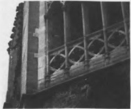
Figure 2. Cracks in buttress of SW pillar of tower.
