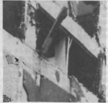
MEXICO CITY: Collapsed infill with columns damaged by "diagonal compression strut."
