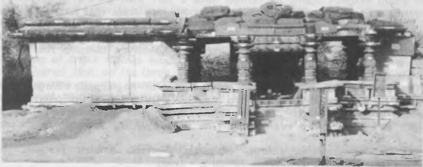
FRONT VIEW OF THE DILAPIDATED TRIPLE SHRINE AT NAGULPAD VILLAGE, ANDHRA PRADESH, INDIA
