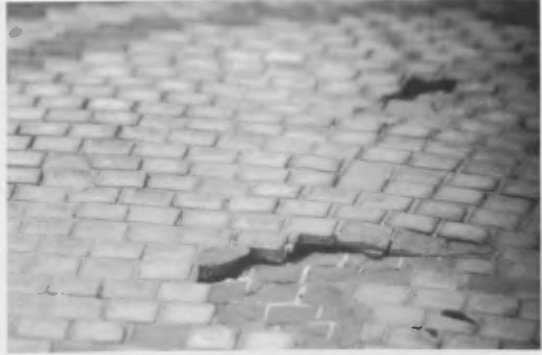
Fig. 3: Deteriorated and delaminated surfaces (photo by Bob Hartzler).
