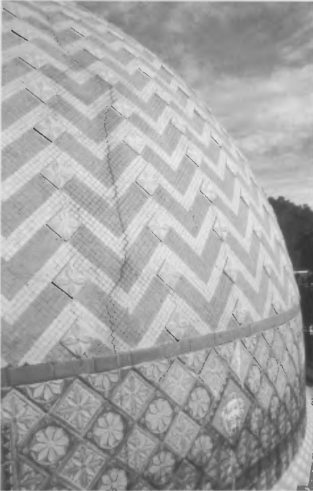
Fig. 1: A section of the Quapaw Dome with a through vertical crack (photo by Jake Barrow).
