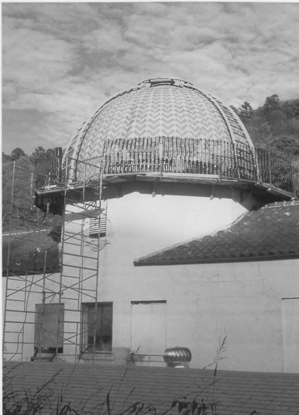
Fig. 6: View of dome with rotating scaffolding in place (photo by Jake Barrow).
