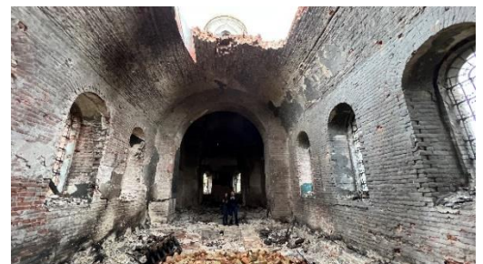
A collapsed vault ceiling of a church in Ukraine. Credits: Aparna Tandon
