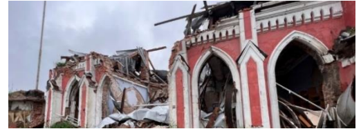
Extensive structural damage to the Regional Library for Children in Chernihiv, Ukraine. Credits: Aparna Tandon
