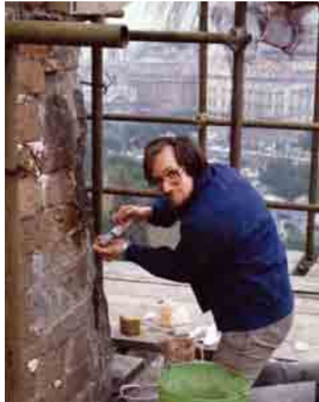
J. Malliet, 1985. As part of the Mortars Research Training Unit (RTU) activities, hydraulic grout was injected into the Campidoglio Towers in Rome.
