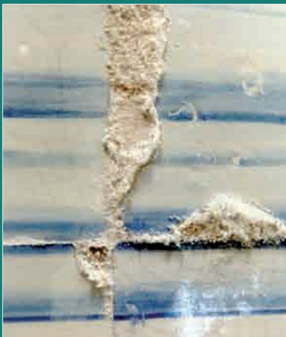
FIGURE 4 Salt efflorescence on joints and glaze lacunae.
