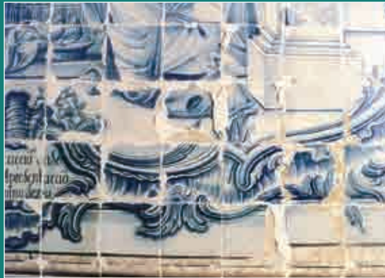
FIGURE 12 Deterioration of the temporary filler after one year.
