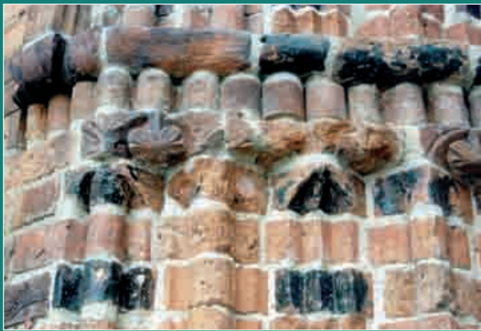
FIGURE 5 (LEFT BOTTOM) Extremely damaged bricks of the St. Jakobi church in Perleberg, Brandenburg, Germany.
