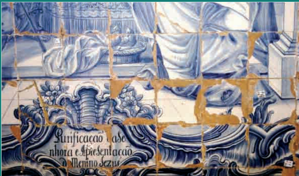
FIGURE 5 Glaze decay caused by salt efflorescence and compression at the joints.
